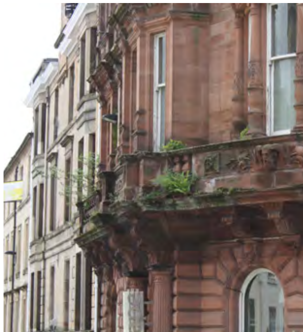
Three quarters of pre-1919 dwellings need repairs to critical elements
